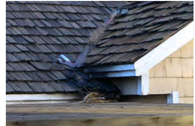
Reducing the structural ignitability of houses, such as replacing wood shake roofs and removing pine needles, is a CWPP objective.
